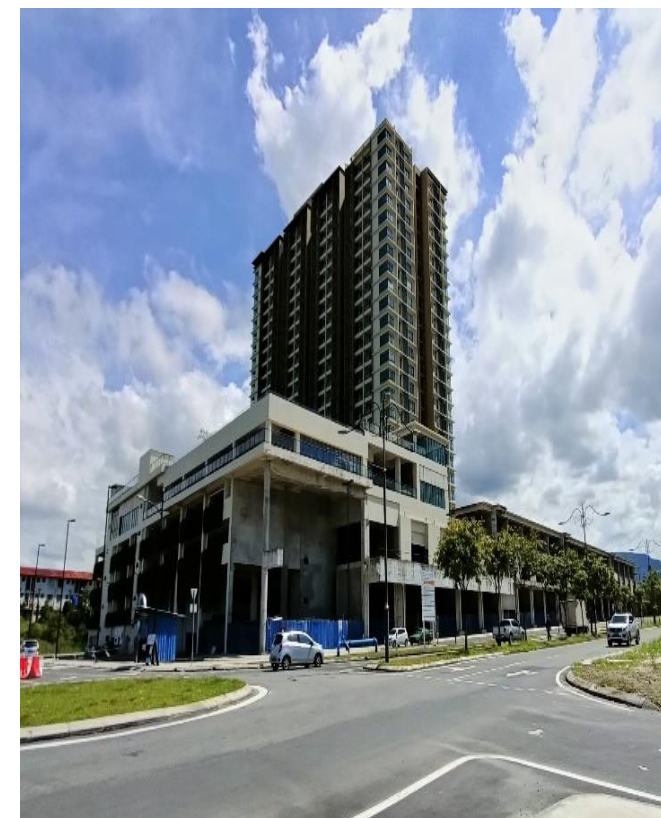
Elemen Utara KK Presint 2 Block A condominium. Pending issuance of Occupation Certificate as of November 2021. Source: WTWS Research
